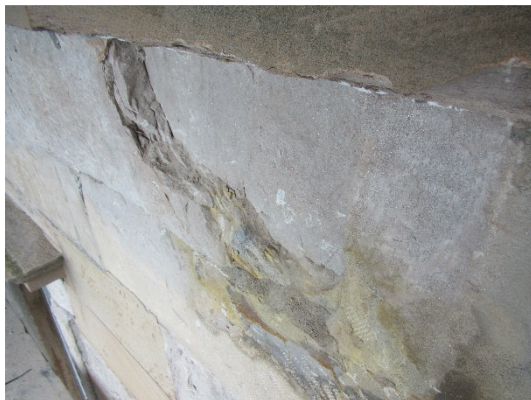
Poor condition of stone
